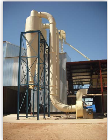
Peanut Drying Plant
